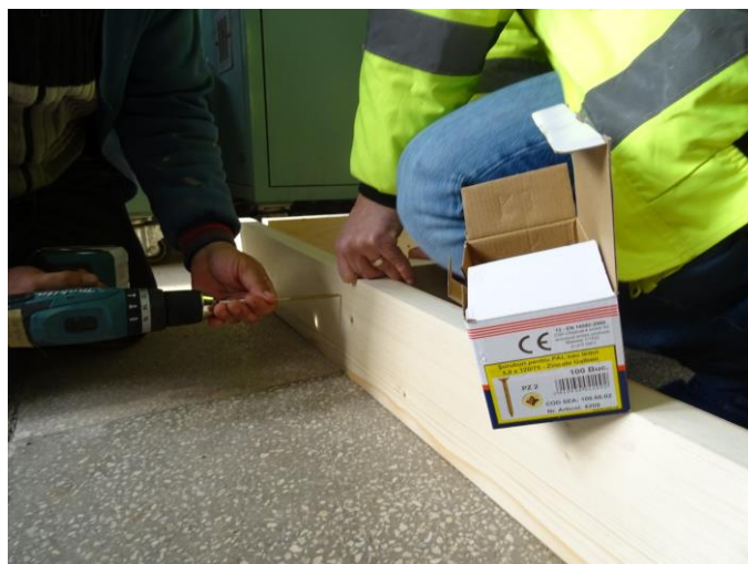
Figure 5 – Connecting the posts with the beams (bottom and upper) by means of screw nails
