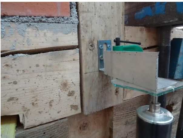
Figure 13: Gap in the connection due to poor execution and superficial crack in the bottom beam
