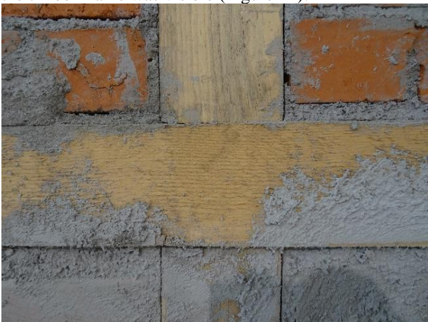
Figure 14: Separation of the masonry infill from the timber frame
