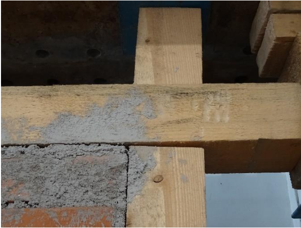
Figure 12: Execution errors: gap in the connections and distortion of the column
