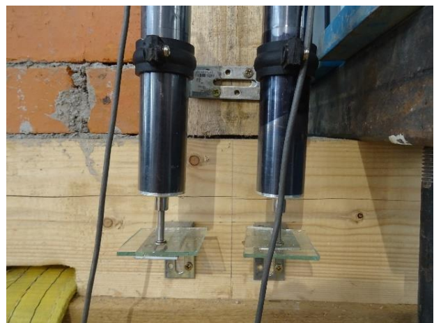
Figure 11: Gap in the connection due to poor execution
