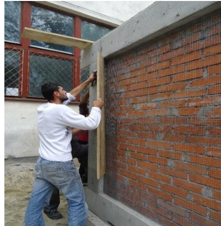
h – bending the wire mesh to follow the shape of the column with a wooden batten
