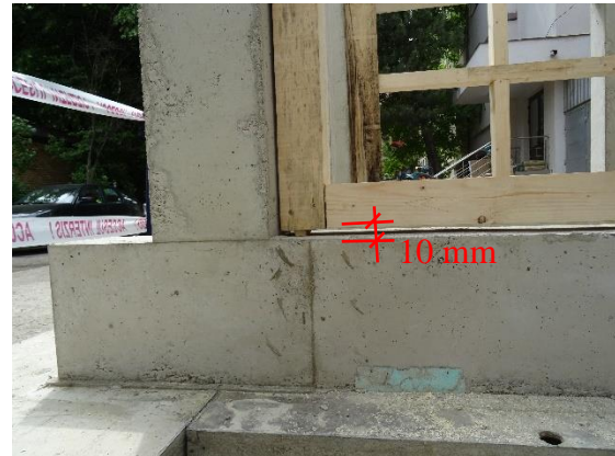
Figure 7. Gap between the RC frame and timber frame, filled with finishing mortar
